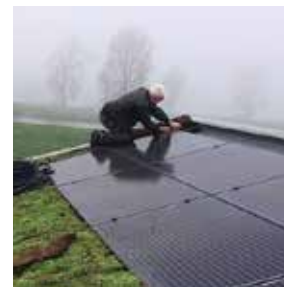
PV-panelen / zonneboiler / ect.
